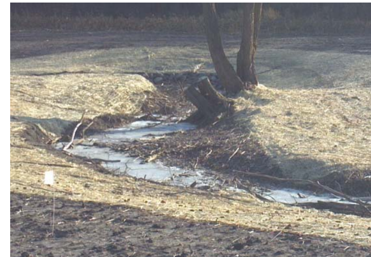
This picture is an example of a BMP recently installed as part of a streambank restoration project along Roy Creek
