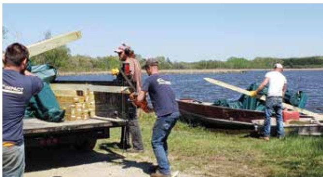
GLSD staff (with assistance from Outdoor Impact) working to install turbidity barrier, May, 2020.
