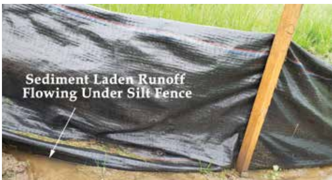
Poor site erosion efforts at a construction site near Green Lake.
